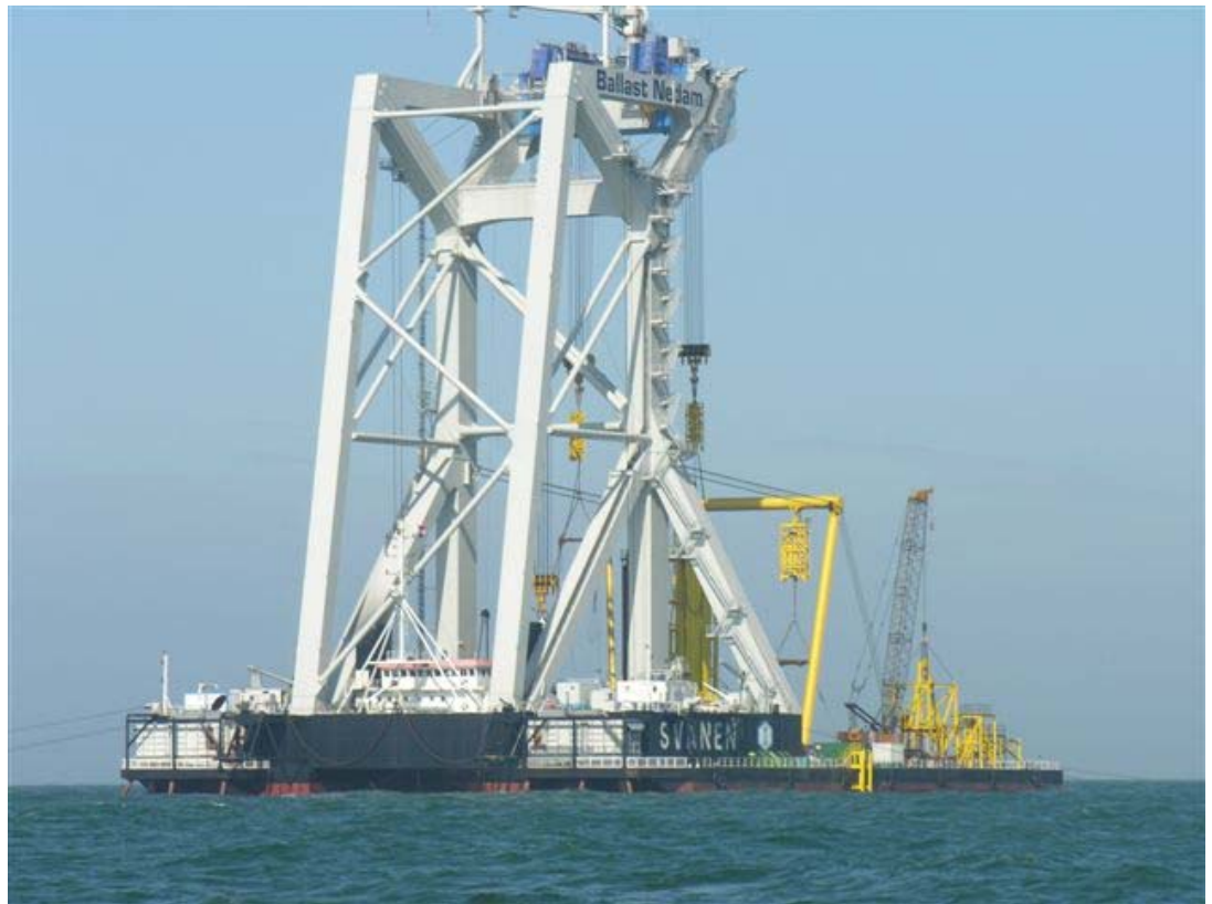
Figure 1. The pile driving ship "Svanen" with its superstructure rising over 100 m above sea level.
